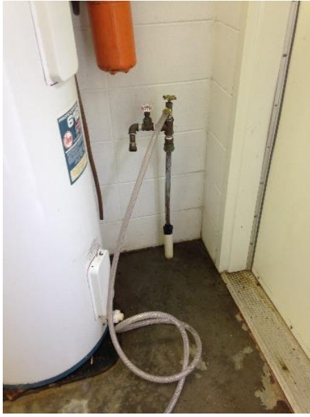
Duteau Creek Headgates Building Raw Water Line Sample Tap Location
