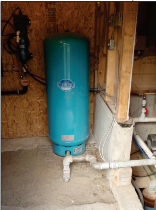
Photo 10: Hydropneumatic tank in the Reservoir Pumpstation.
