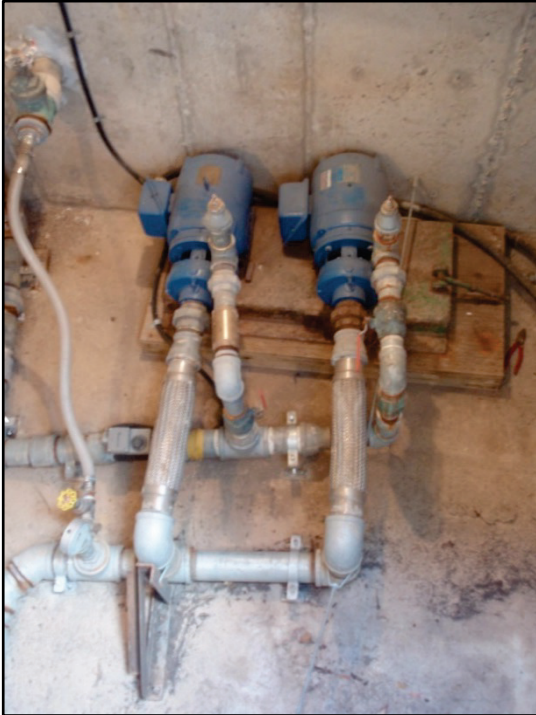
Photo 5: Lake Pumpstation pumps.
