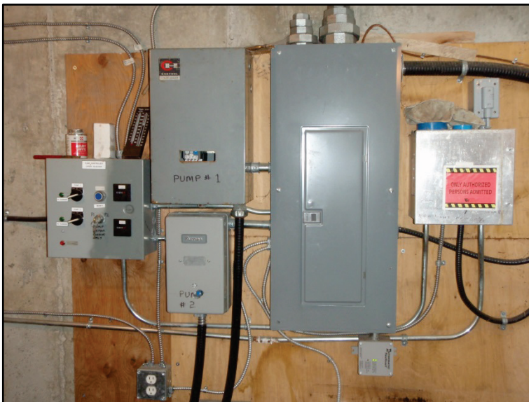
Photo 6: Lake Pumpstation electrical (in the chamber).
