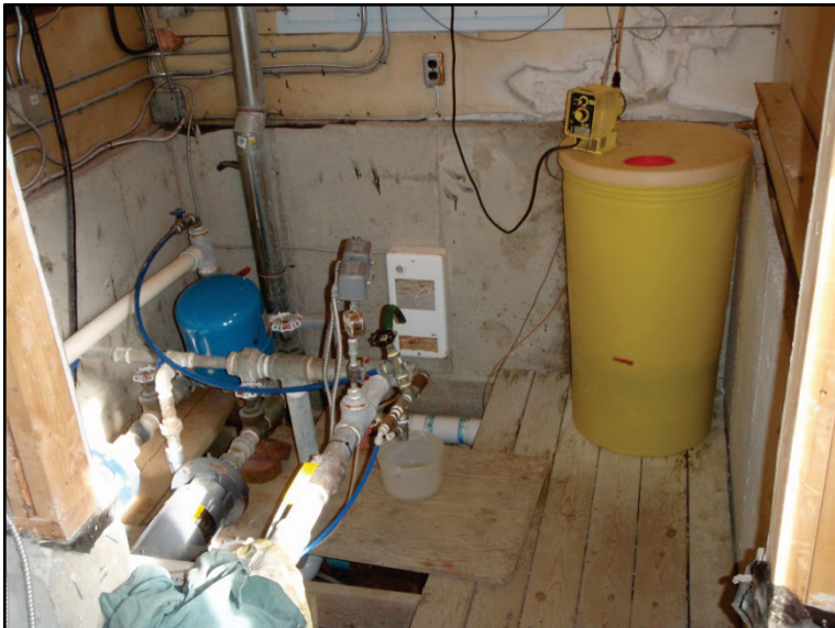
Photo 8: Reservoir Pumpstation including chlorine injection equipment.
