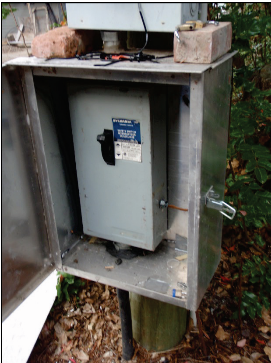
Photo 4: Lake Pumpstation emergency electrical cut-off switch located outside of the pump chamber.
