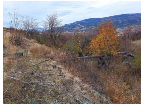
Figure 12: View northeast of discharge pipe/spillway of canal into riparian gully feature connecting to Wetland 5
