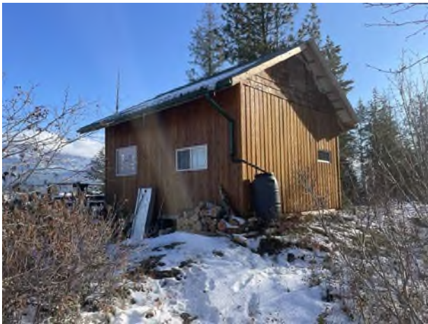
Firewood stacked against the building.
