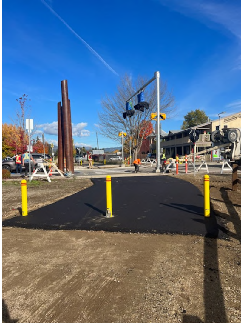
Caption: Construction crews finalizing a crossing for the Shuswap North Rail Trail in Enderby, BC.
